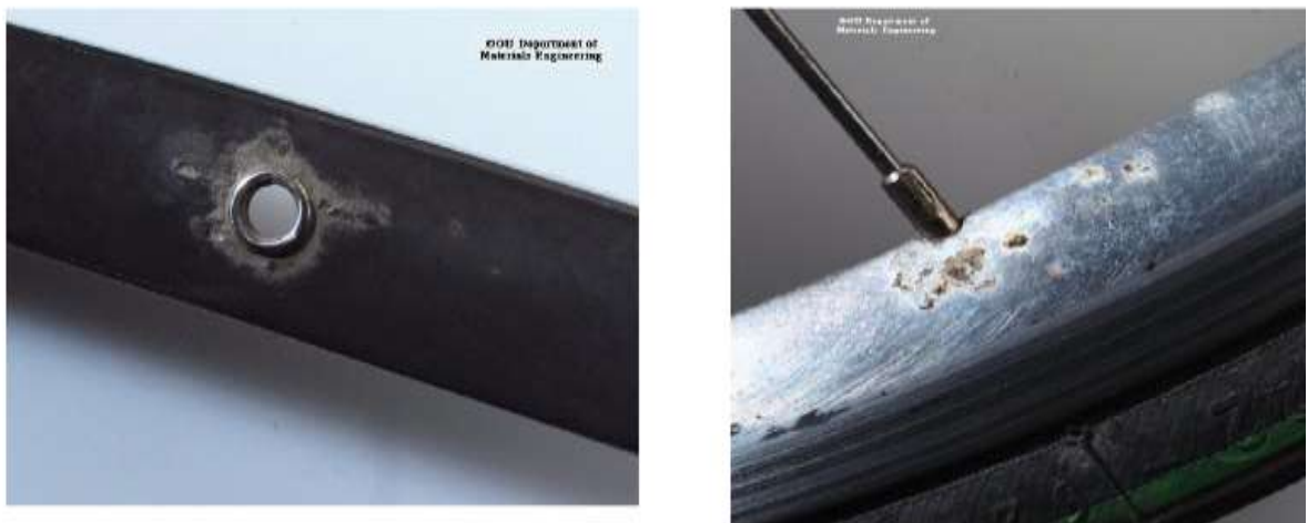
Figure 5. 17 Indirect corrosion "Galvanic corrosion"
