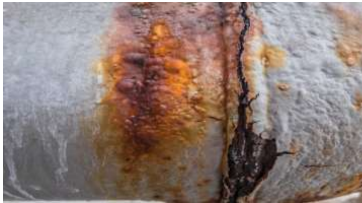
Figure 5. 18 Stress corrosion cracking
